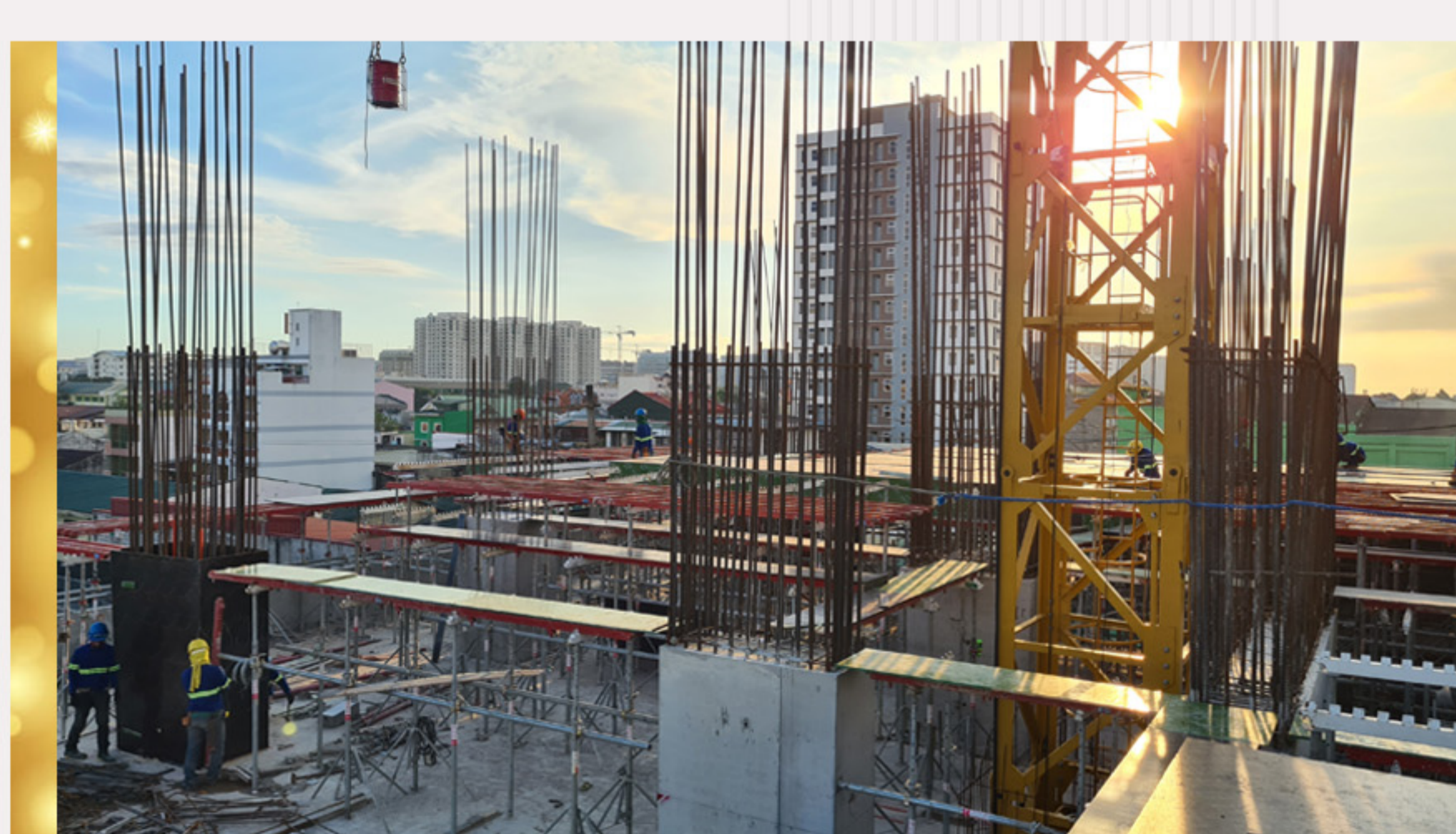
Formworks installation for beams and girders (5th floor- Zone 4) 五層樑柱模板安裝 (4區)
