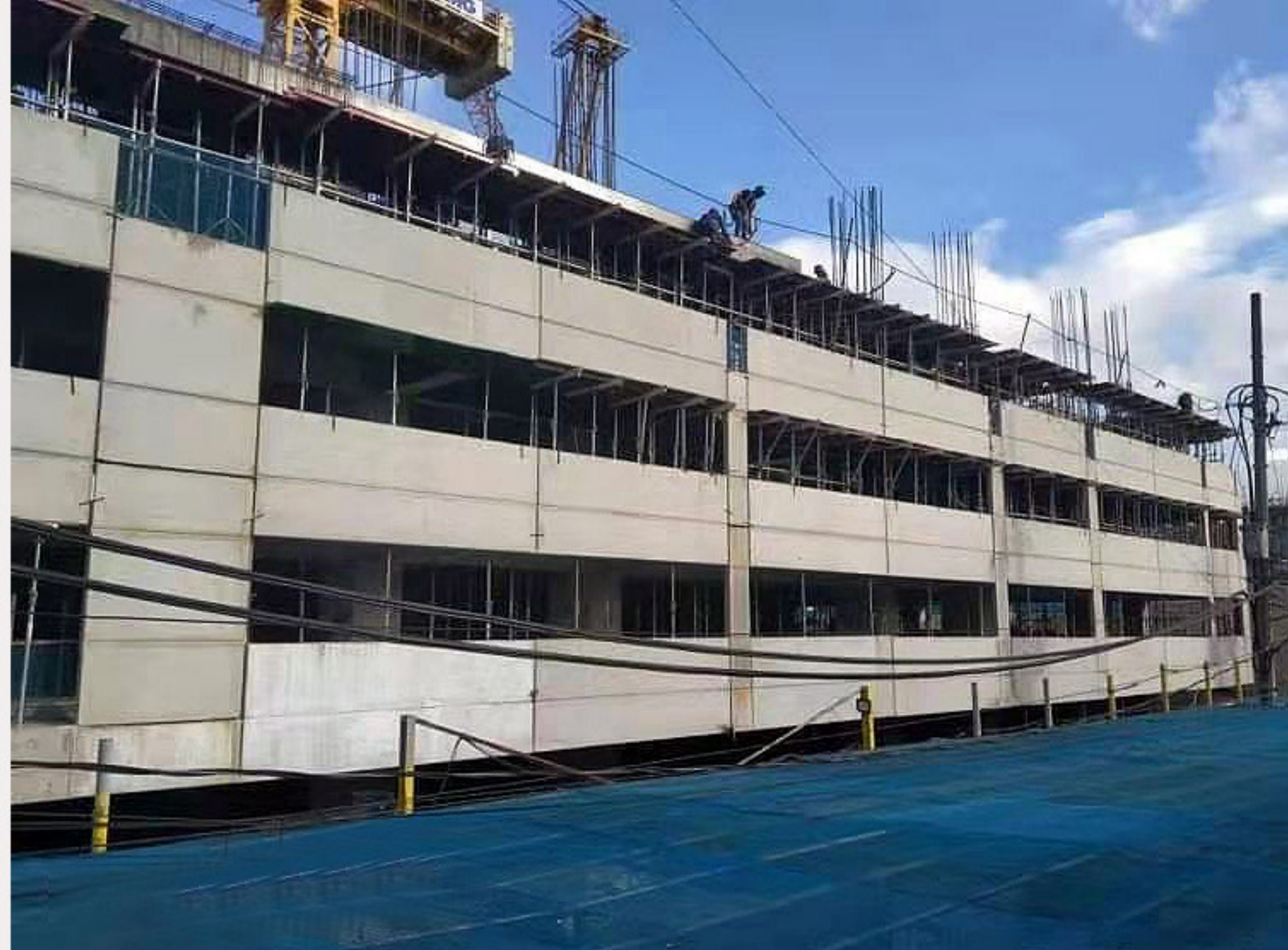
Left side front (installed precast wall @4th floor) 停車場外牆已安裝至四層
