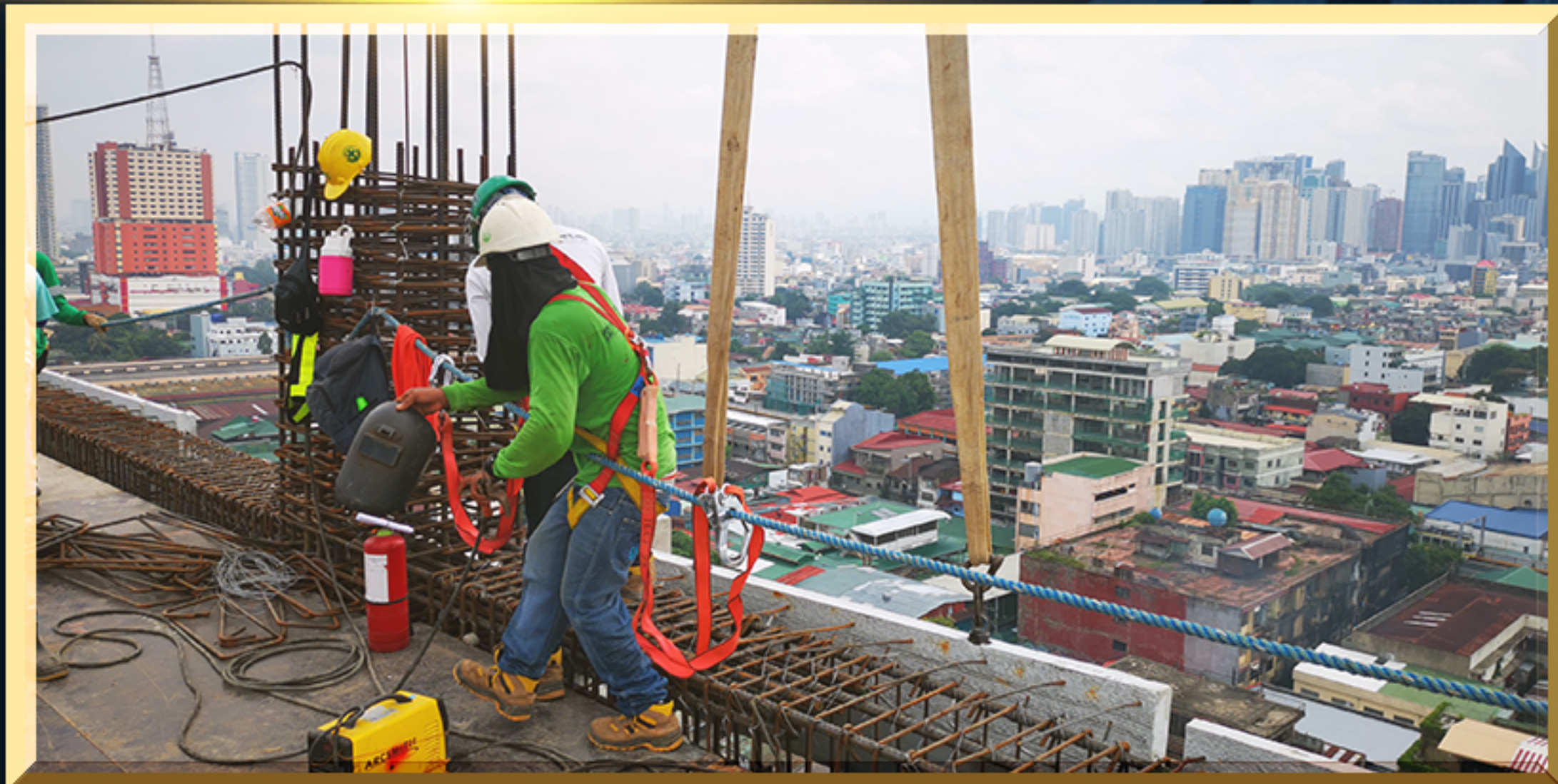
Installation of Precast Wall (17th Floor, Zone 2 and 4) 第17樓2區和4區外牆預製板安裝
