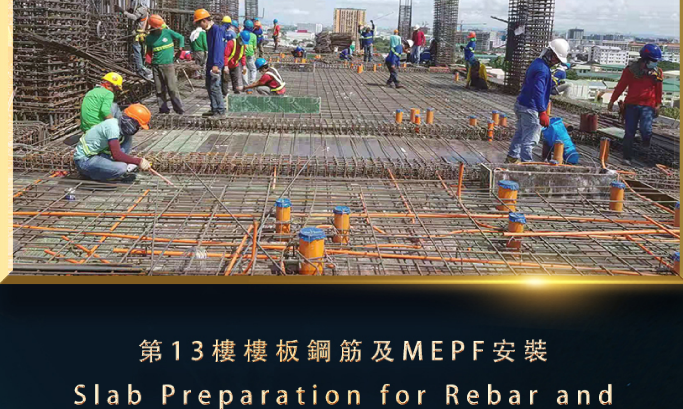
第13樓樓板鋼筋及MEPF安裝 Slab Preparation for Rebar and MEPF works (13th Floor)
