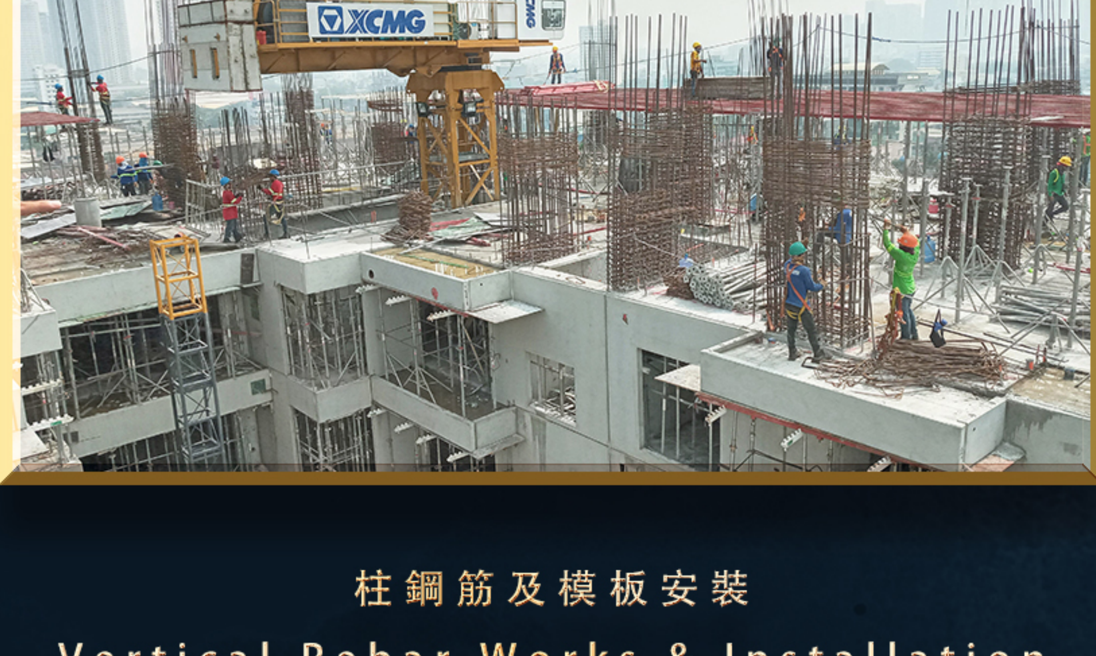
柱鋼筋及模板安裝 Vertical Rebar Works & Installation of Props for Formworks
